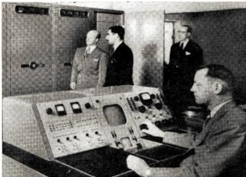
ARGENTINA's first TV station, LR-3-TV Buenos Aires, on Channel 7 has been fully equipped by Federal Telecommunications Labs., subsidiary of IT&T. Shown here is the transmitter room of the 45 kw installation on the 24th floor of the Ministry of Public Works Bldg. Standing in front of the transmitter are (l to r): J. M. Valentine, FTL engineer in charge of the installation; J. C. Coriat, Standard Electric Argentina, IT&T subsidiary; H. L. Johnson, FTL. Station technician at control console is not identified.
